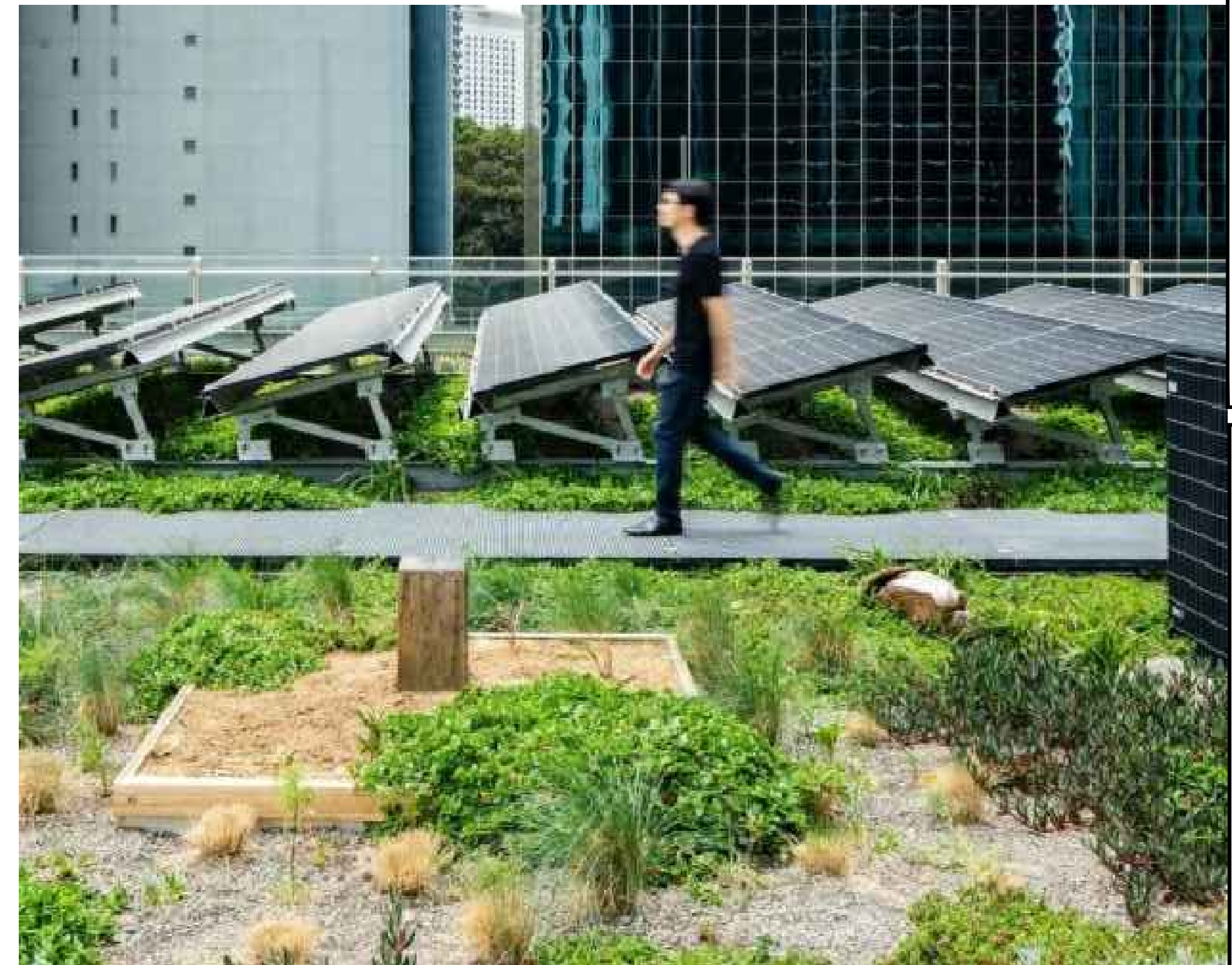
GREEN ROOF & SOLAR PANELS
